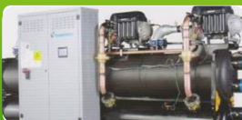
Oil-free Chiller (4 out of 12 installed) - 40M baht
