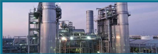
Amata Power Plant 5 blocks : 734 MW
