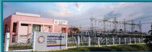
Power Substation of PEA 3 Substations : 300 MW
