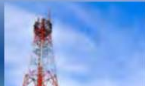
Solar for Tower Co System
