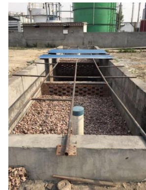
Rainwater harvesting system
